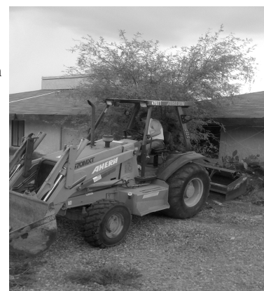
Over five years of growth, weeds and dead bushes were removed cleaning up the outside of the buildings.
